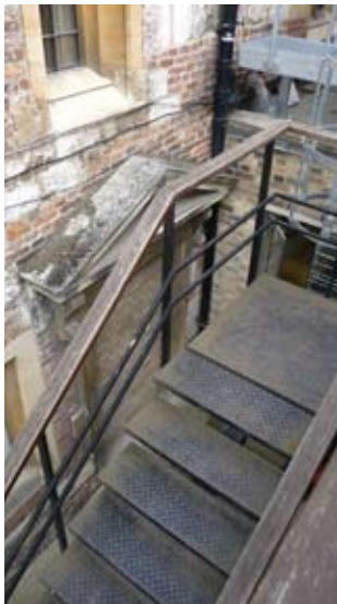
Fire escape compromises library court and blocked up historic doorway
