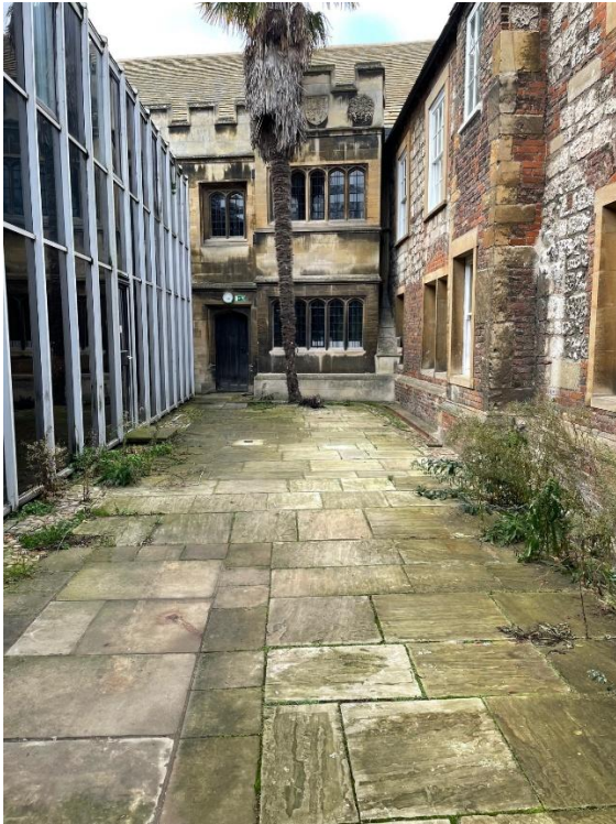
From left to right, the present library, the Bodley Library and First Court (south elevation) showing the proximities and poor quality of space.
